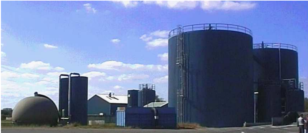
Figure 4 Co-digestion facility for food, manure and other wastes in Denmark – biogas holder left; two digesters right with the two 70 °C sanitisation towers in their shadow.
